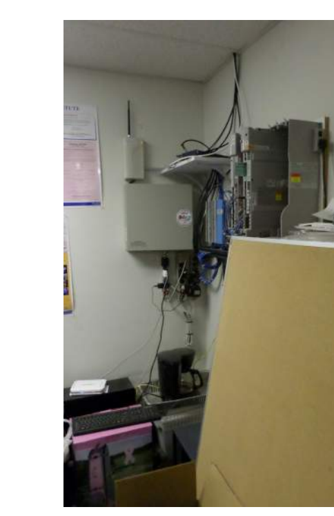
VIEW OF DATA PANEL.
