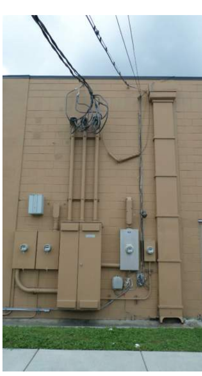
ELECTRICAL METERS @ REAR OF BLDG. 3
