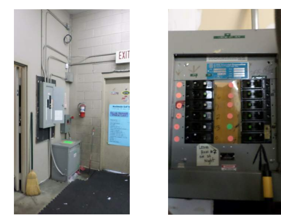
VIEWS OF ELECTRICAL PANELS.
