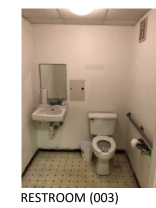
1 RESTROOM COMPLIANCE (PHOTOS) NOT TO SCALE
