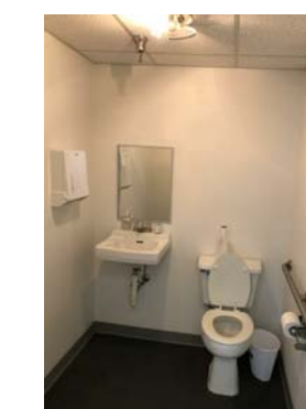
1 RESTROOM COMPLIANCE (PHOTOS) NOT TO SCALE
