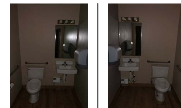
1 RESTROOM COMPLIANCE (PHOTOS) NOT TO SCALE
